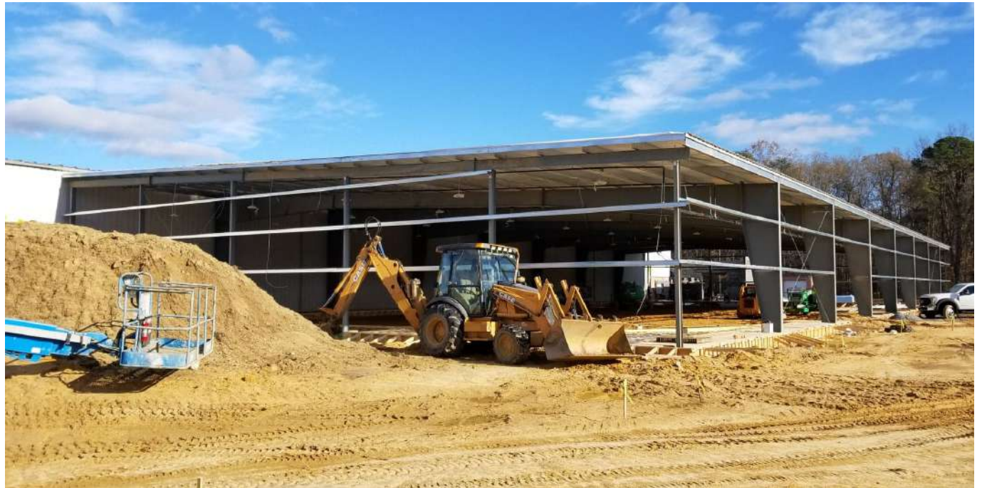
Construction of the long-planned second sheet of ice at Piney Orchard Ice Arena is well underway. It is slated for completion this winter.
